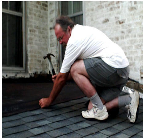
John Graham spent most of July and August installing new roofs to winterize the house.
